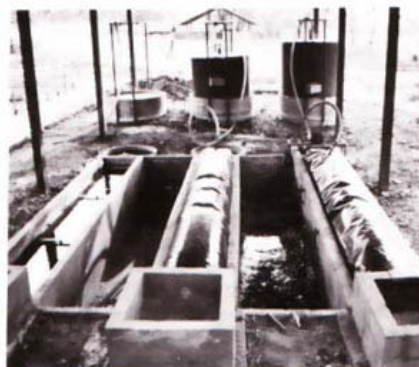
AIT-designed plug flow digesters installed at the Tabkwong Swine Research Station.
