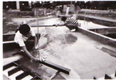
Model study of Lower Mae Ping project, pump storage of Bhumibol Dam.
