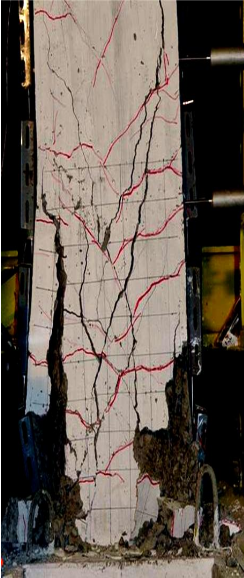
Picture 2a: (left) Reinforced column after subjected to earthquake-induced cyclic loads
