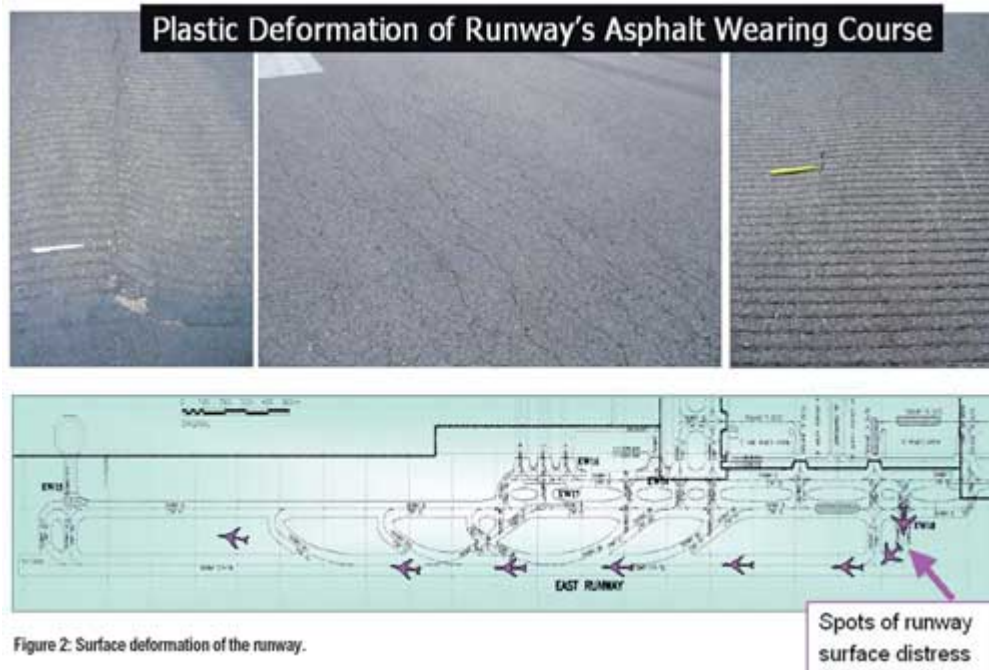
Figure 2: Surface deformation of the runway.
