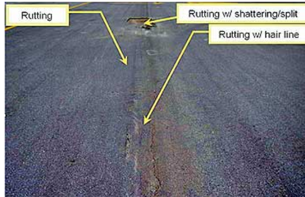
Figure 1: Typical distress in the taxiways and taxilanes.
